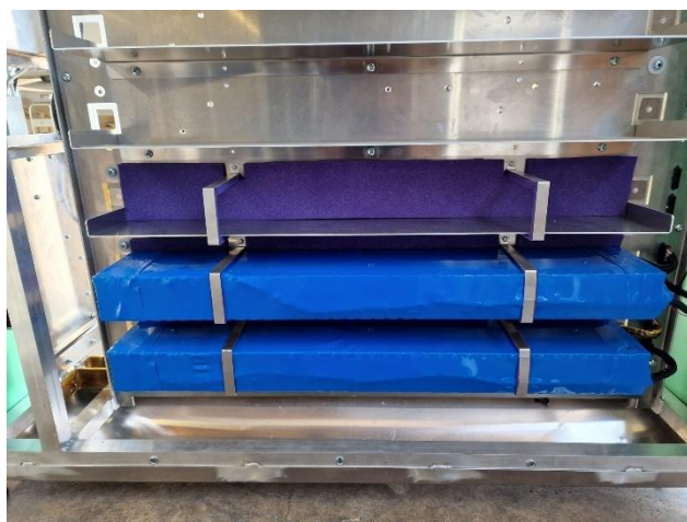
Figure 44 The modules inside the battery
