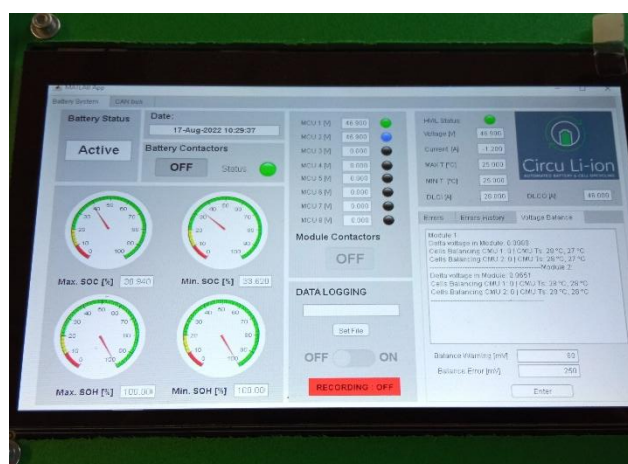
Figure 45 The battery HMI
