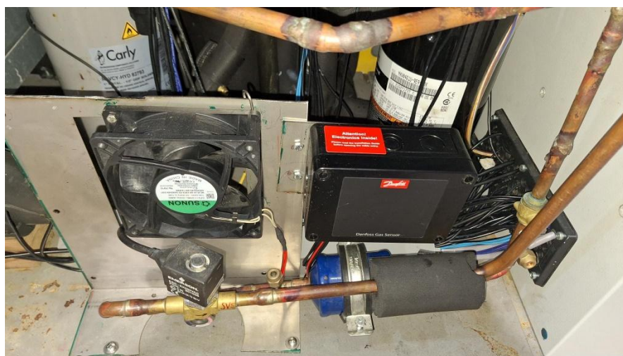
Figure 29 Leak detection sensor and extraction fan
