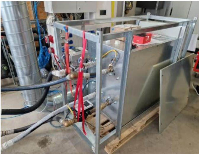
Figure 6 Hydraulic connection of R290 35kW BW-HP on test bench
